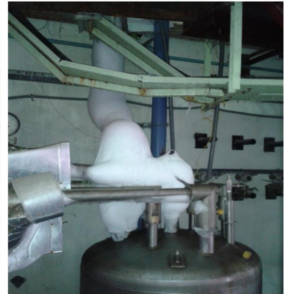
Frosting on vent line
