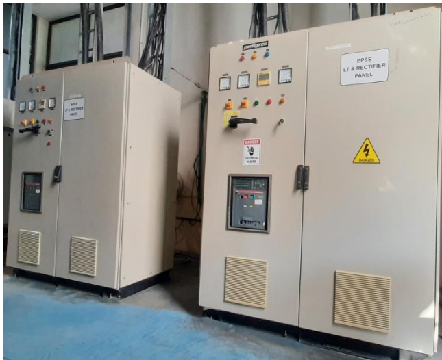
Rectifier section of 11kV 35A and 35kV 15A DC Power supplies installed at IPR
