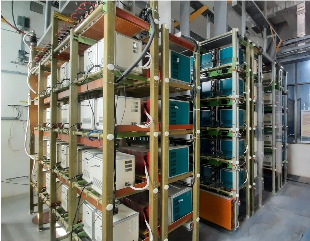
Module section of 11kV 35A and 35kV 15A DC Power supplies installed at IPR
