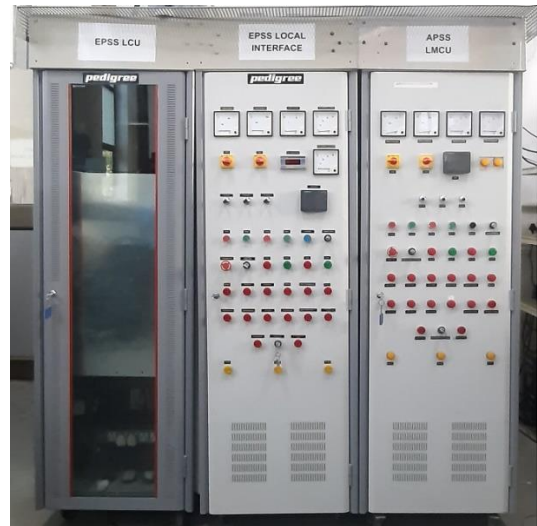
Control section of 11kV 35A and 35kV 15A DC Power supplies installed at IPR
