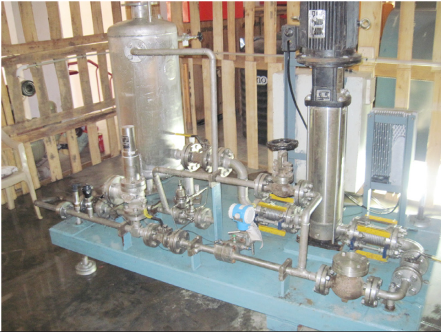
Figure A.2.2.2 Portable Water Circulation System (100 LPM, 80C, 20 bar) assembly prior to thermal insulation.
