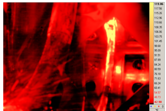
Figure A.1.1.4.8. Infrared image of the Aditya limiter
