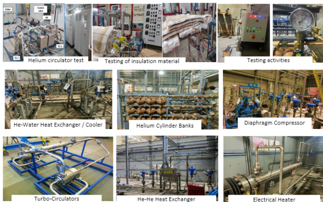
Figure A.4.5: Major components of the EHCL system installed, integrated and tested at site.
