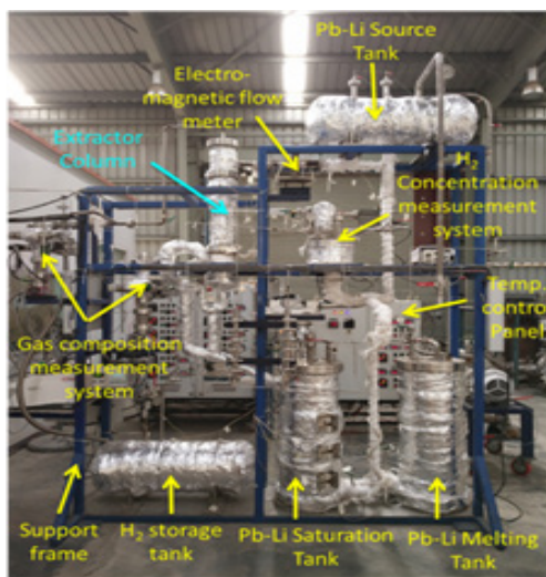
Figure A.4.12: Installed HIES set-up.
