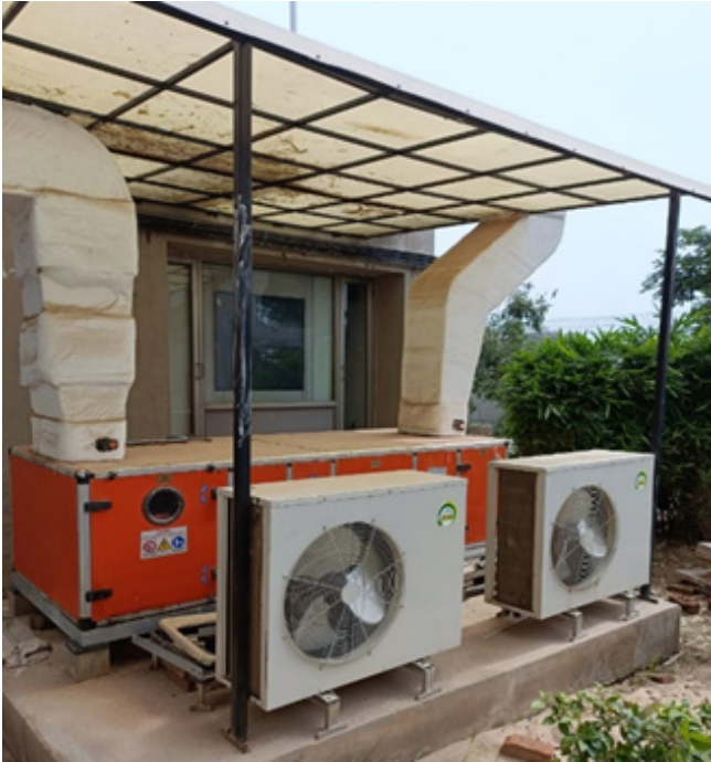
Figure D.2: Direct expansion air handling unit and air conditioning system is for existing class 10000 clean room for SRP Lab at FCIPT campus.
