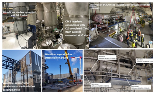
Figure B.1.5: Installation of X, Y cryolines and warmlines at ITER site.
