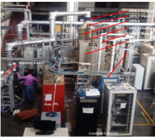
Figure A.3.10: View of Installed RF source in SST-1 hall.
