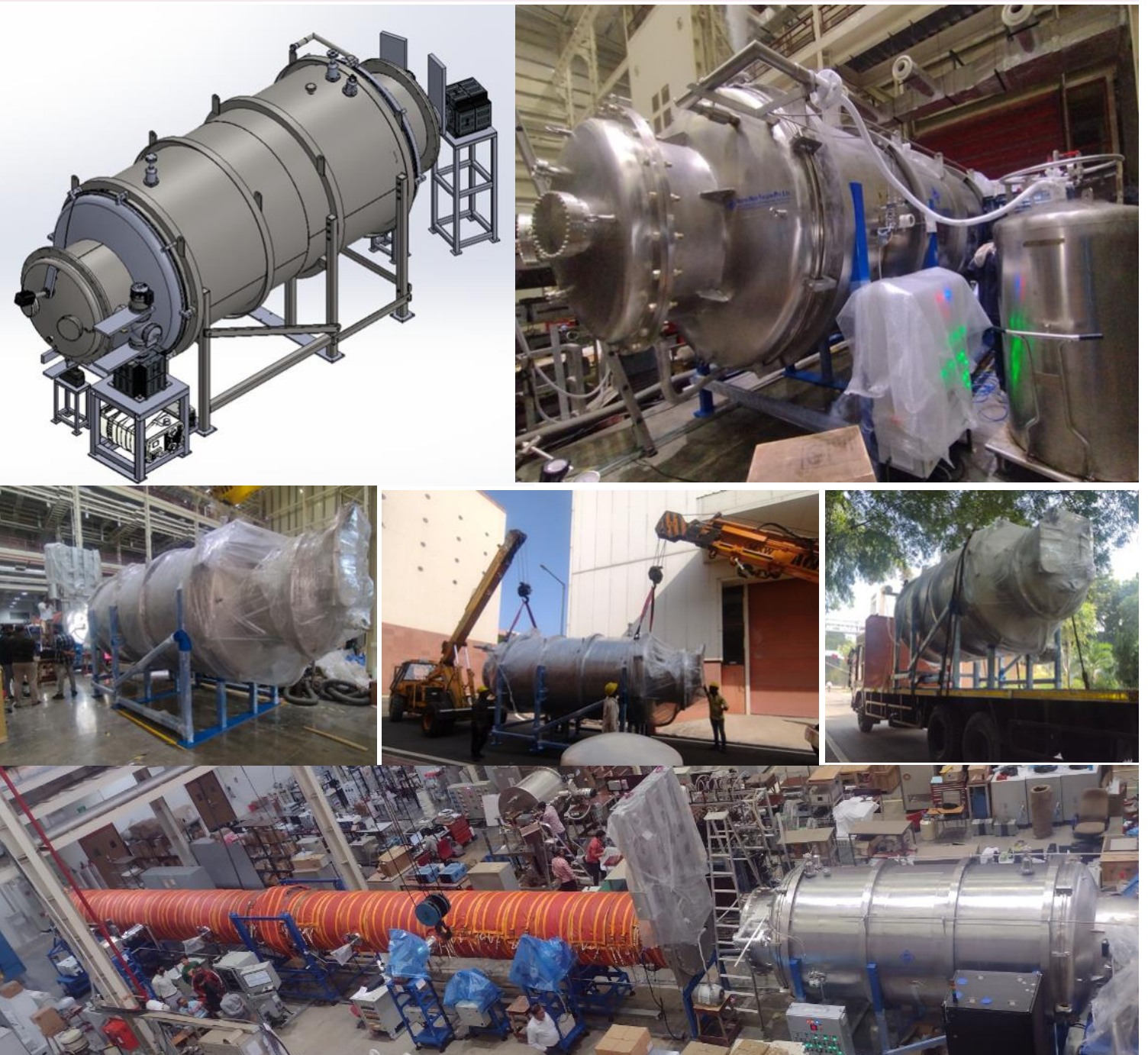
Images of the installation of the cryo-pump for the LIGO-India VISTA facility at IPR
