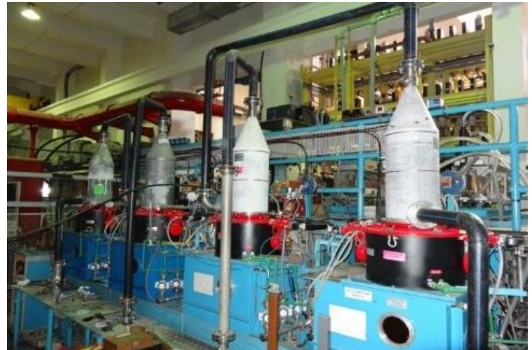
Figure-2: HP LHCD source system, comprising of four klystrons, each rated for 0.5MW-CW RF power at 3.7 GHz
