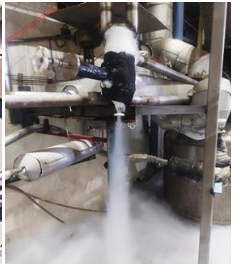
LN 2 outlet at Sub-cooler vessel
