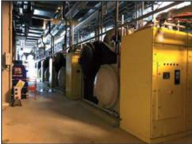
Figure B.1.5: Water cooled chillers.
