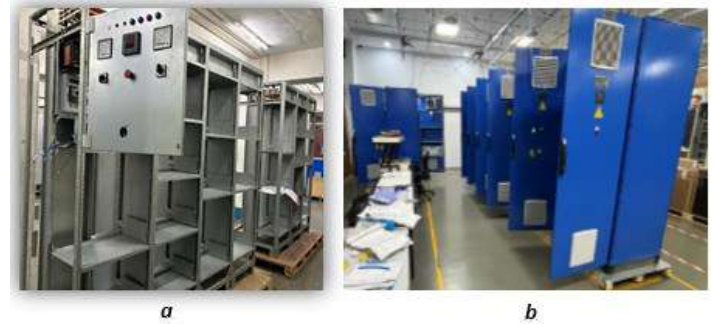
Figure B.1.12: I&C cubicles.
