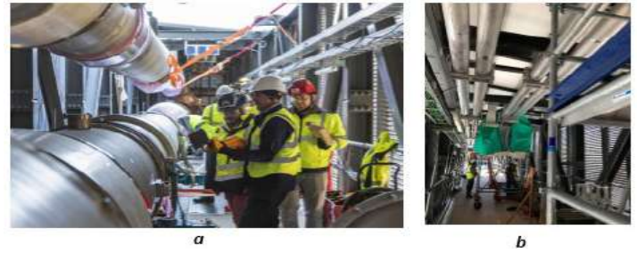
Figure B.1.11: Installed Cryolines at ITER site.
